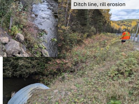
Ditch line, rill erosion
