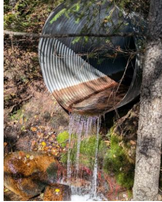
Hanging Culvert & undercut
