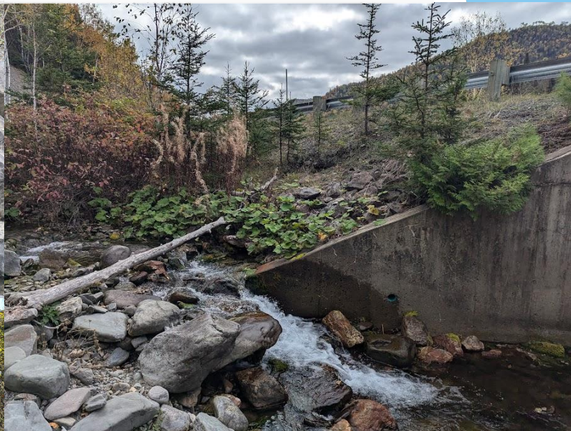
Culvert Scouring & Undersized Culvert
